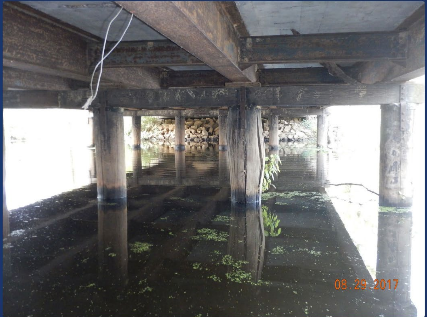
Timber pile with large bulge in the middle and many vertical cracks. Timber cap shows no signs of deterioration or overstress.
